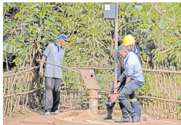
Mr. Niyonteze Sepiriyo, a resident of Ssenda Kakindu in Mityana district observes technicians from Whave Solutions as they carry out repairs on a borehole.
